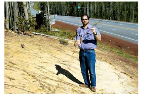
Figure 3-50 | Wind erosion removes topsoil and exposes roots
