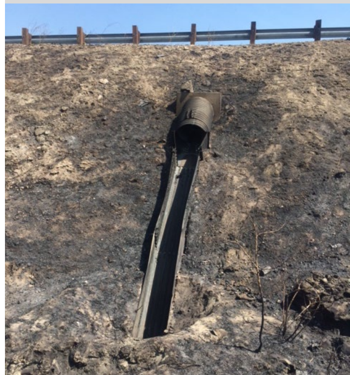
Culverts and drainage structures can also be damaged by roadside fires and have to be inspected after a fire. The extent of unvegetated loose soil along the roadside embankment shows the potential for serious erosion problems after a roadside fire.
