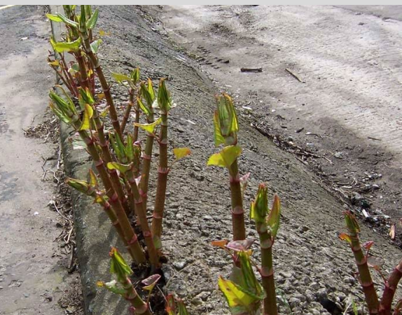
Japanese knotweed growing along a reinforced embankment
