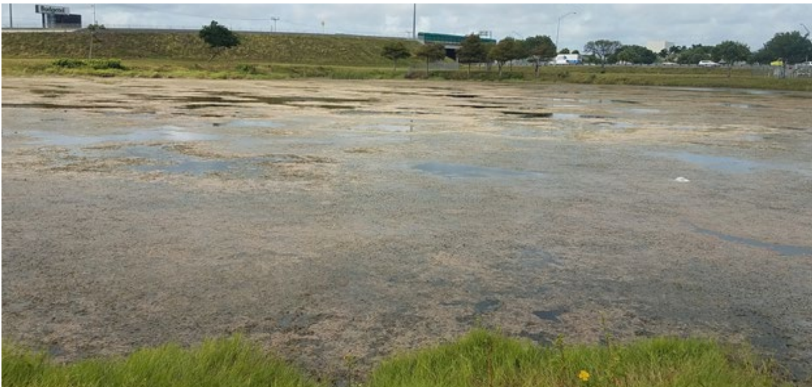
A stormwater pond that captures stormwater from the Florida Turnpike filled with hydrilla.
