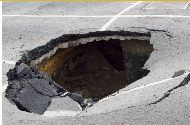
Above is an example of the type of damage that can occur from an iguana burrow beneath pavement.
