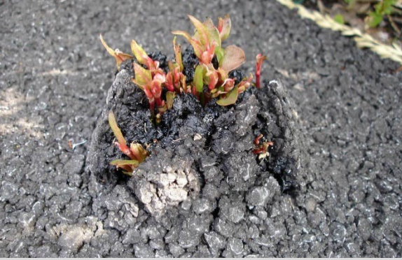
Japanese knotweed growing up through pavement.
