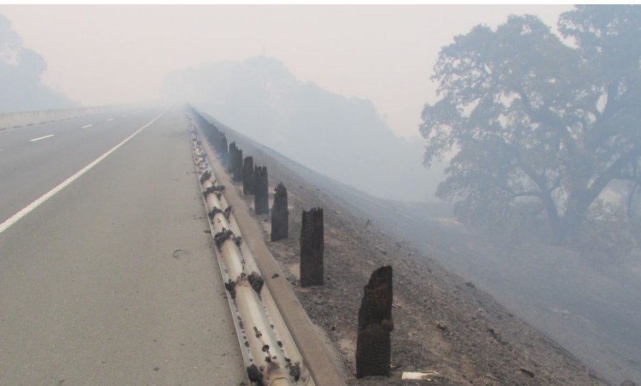
Burnt guardrail posts and unvegetated, loose soil susceptible to erosion.
