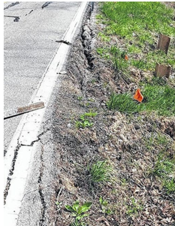
Roadside embankment erosion can cause pavement cracking.
