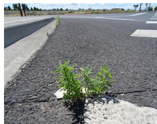
Kochia growing in pavement seam and edge of pavement.
