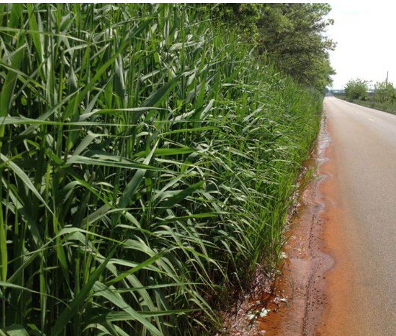
The density of phragmites prevents water from draining off roads causing flooding in roadway and in the winter creating dangerous ice buildup.
