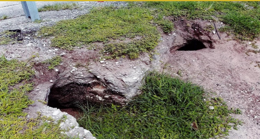
Two large green iguana burrows along the Florida Turnpike in south Florida. These large burrow entrances are right at the edge of pavement. The burrows likely extend beneath the roadway and could cause the roadway to collapse. These areas have to be repaired as quickly as possible.
